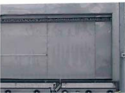
High-pressure washing plant
